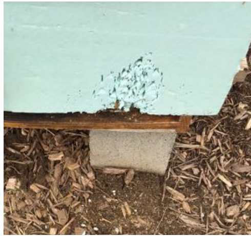
Damage to the insulation
